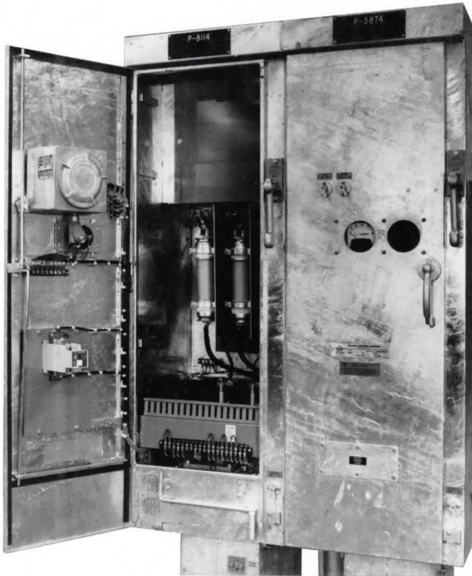
CONTROLLER WITH CABINET DOOR OPEN & DOOR CLOSED
