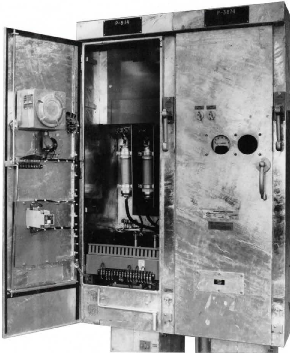
CONTROLLER WITH CABINET DOOR OPEN & DOOR CLOSED
